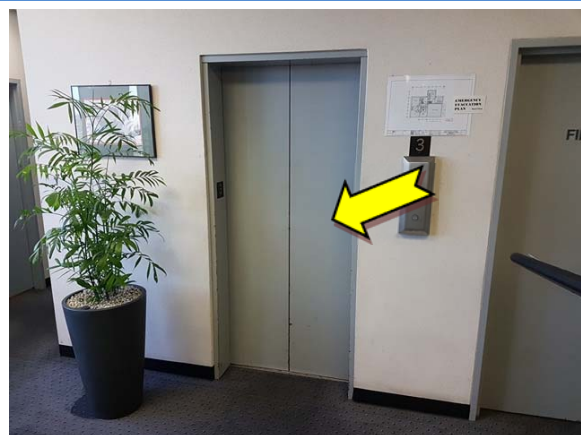
Photo 12. Interior, level 3, lift doors – suspected asbestos-containing insulation door core.
