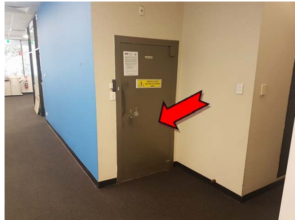
Photo 16. Interior, ground level, strong room, door – suspected asbestos-containing insulating door core.
