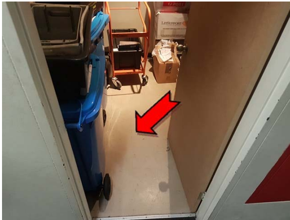
Photo 15. Interior, ground level, central store room, beige floor coverings – assumed asbestos-containing vinyl floor tiles.
