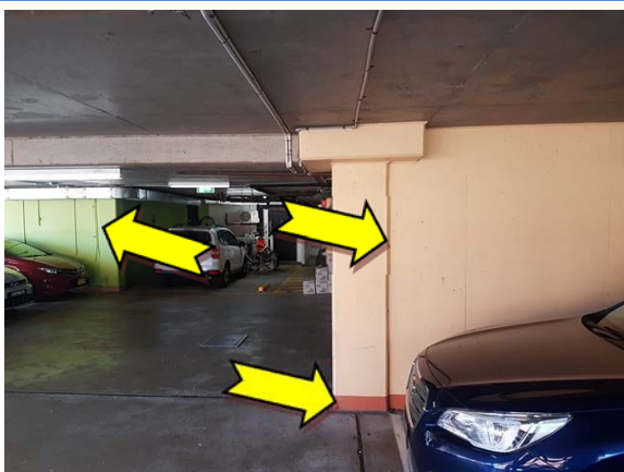
Photo 23. Interior, basement level, car park, walls – suspected green, light orange and dark orange upper coloured paint systems.
