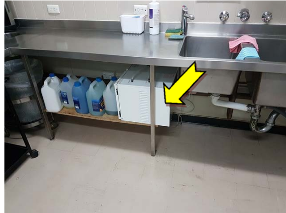
Photo 20. Interior, level 3, kitchen, hot water boiler – suspected SMF internal insulation material.
