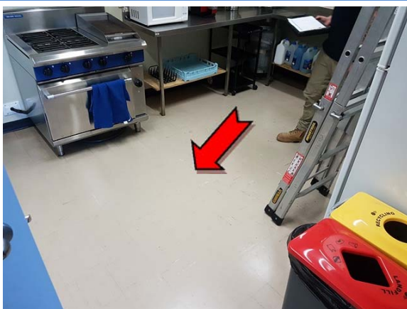
Photo 11. Interior, level 3, kitchen, floor coverings – assumed asbestos-containing beige vinyl floor tiles.
