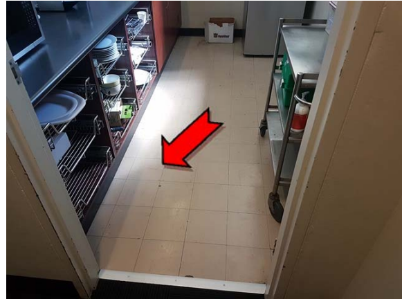
Photo 14. Interior, level 1, kitchen, north-east, beige floor coverings – assumed asbestos-containing vinyl floor tiles.
