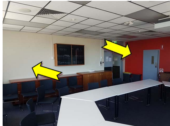
Photo 22. Interior, throughout, wall – suspected lead-containing red and cream upper coloured paint system.
