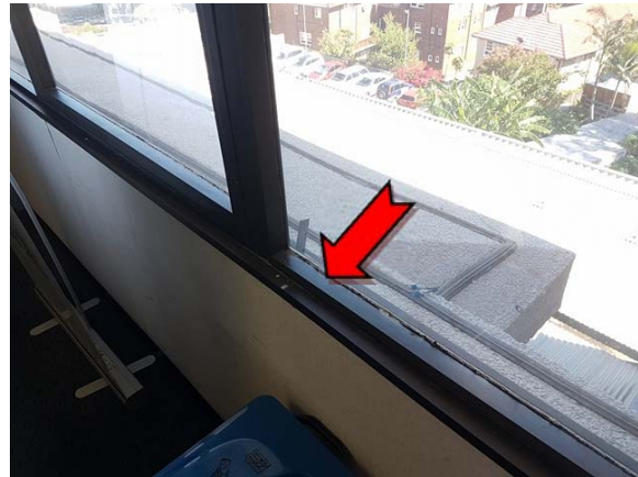
Photo 10. Interior, level 3, lift lobby, window frames – asbestos-containing window caulking.
