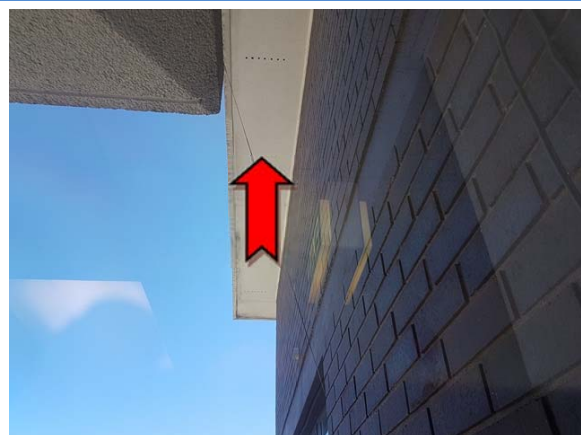
Photo 6. Exterior, throughout, eaves – suspected asbestos-containing fibre cement sheeting.
