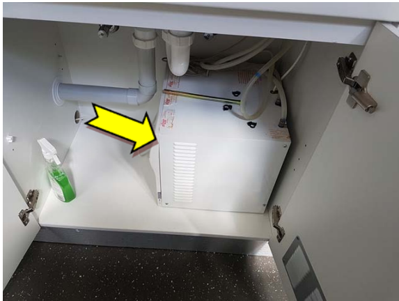
Photo 21. Interior, level 2, north-west, kitchen, hot water boiler – suspected SMF internal insulation material.
