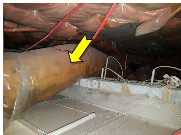
Photo 18. Interior, throughout, ceiling space, flexible ductwork – suspected SMF internal insulation material.
