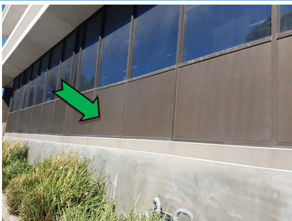
Photo 5. Exterior, throughout, infill panels – non asbestos-containing fibre cement sheeting and suspected lead-containing brown upper paint systems.
