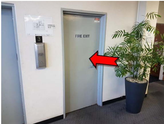
Photo 9. Interior, all levels, fire doors – suspected asbestos-containing fire door cores.
